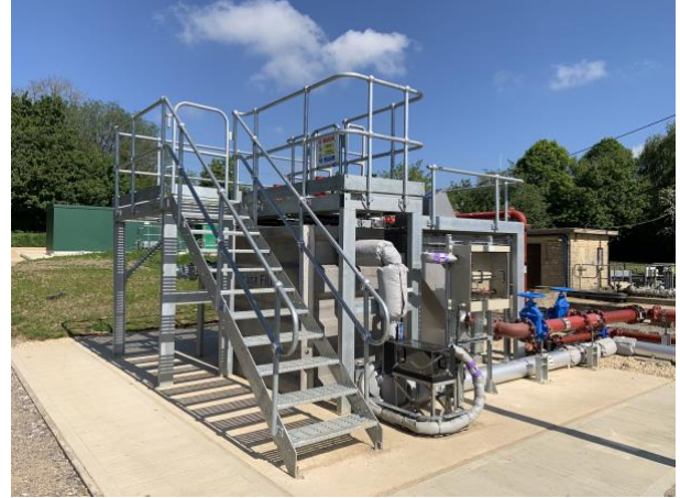
Eydon STW • TF6 Drum Filter
