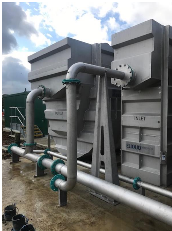
Stewkley STW • SF2/10-disc Filter Unit with Floc Tank
