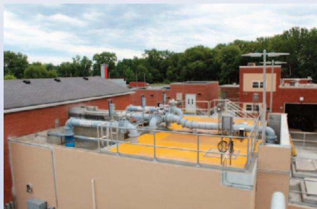
A concrete built Pile Cloth Media Primary Filtration system operating at a municipality for primary treatment.
